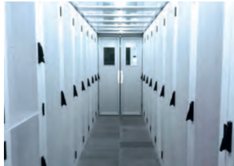
DATA CENTER SWISSCOM | GUENIN ATELIER (2014_Lausanne)
