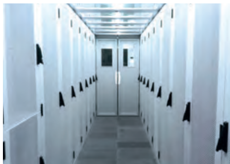
DATA CENTER SWISSCOM | GUENIN ATELIER (2014_Lausanne)
